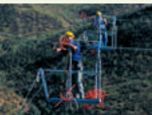
Marking of lines with spiral devices "bird flight diverters".
