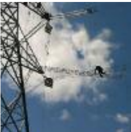
Power cables L/Castejón-Muruarte.
