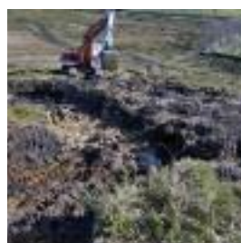
Photographs 2 and 3. Moving of habitat substrate of protected amphibians and plant species in the area which crossed the work area of
