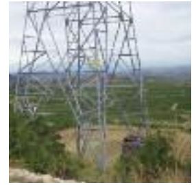
Junction support for the power line from the SS. Haro
